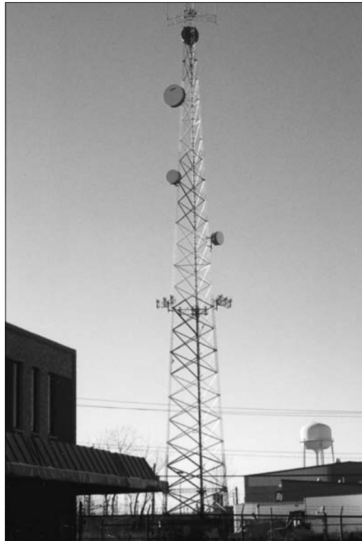
Figure 3-11 A typical microwave tower and antenna
