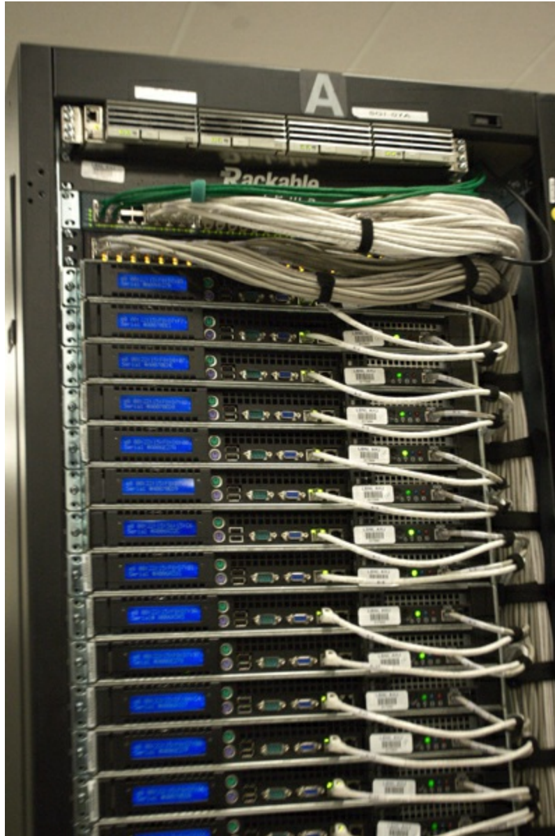
Figure 3.28. Rack of commodity servers Photo by D Coetzee / CC BY 1.0
