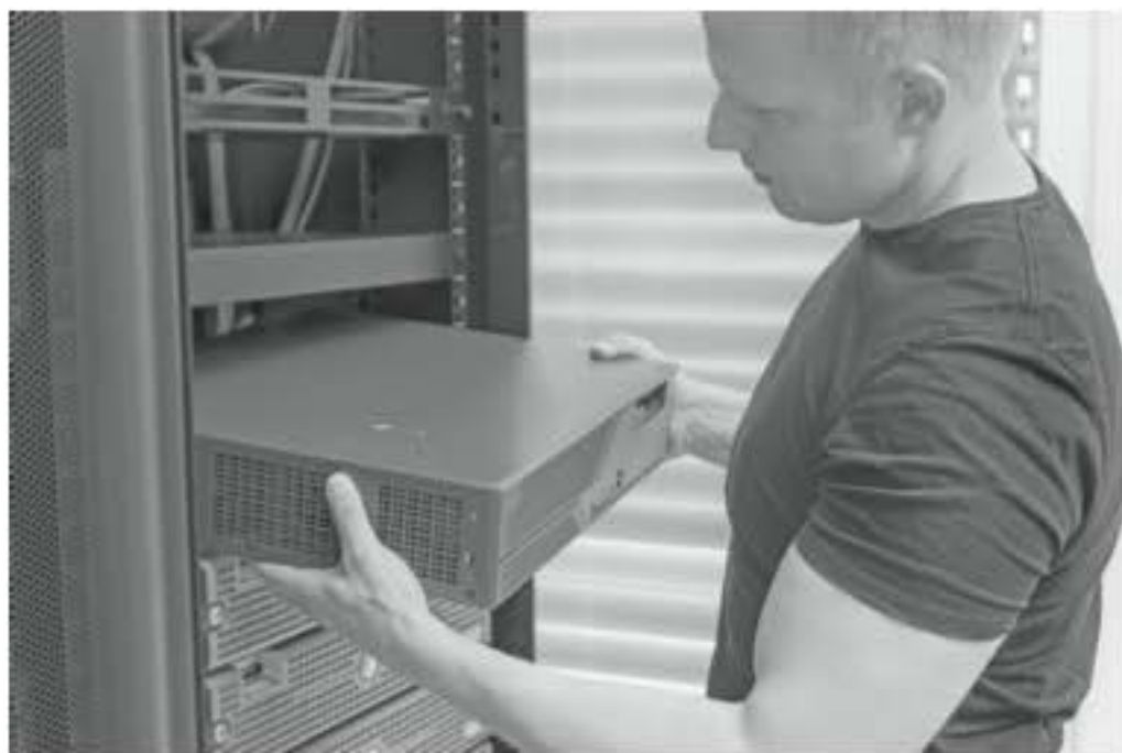
FIGURE A-27 Rack Server
