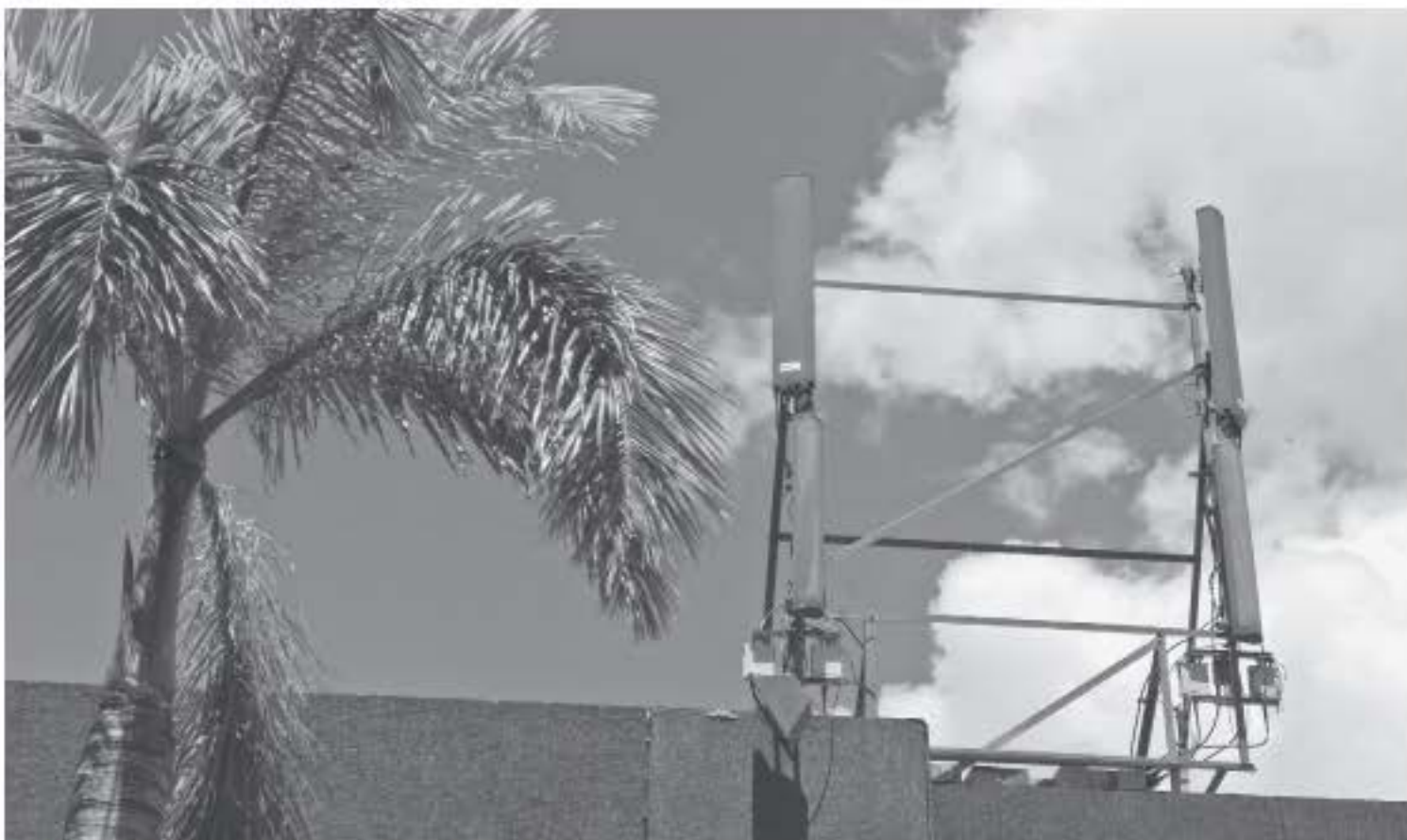
FIGURE 10-9 Cellsite with Paddle Antennas
