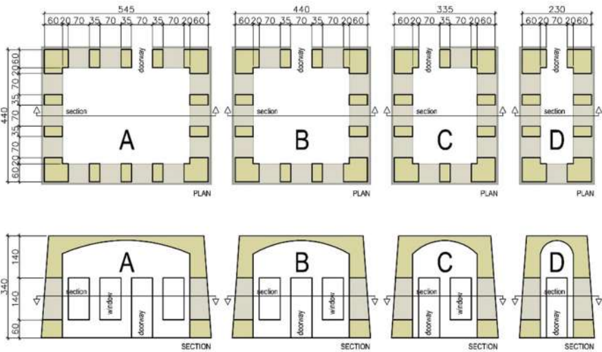
Fig. 2. Typical plans and sections of single floor cas house modules in different sizes varying according to the number of the façade openings.
